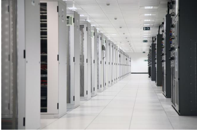
Figure 1: A data centre
