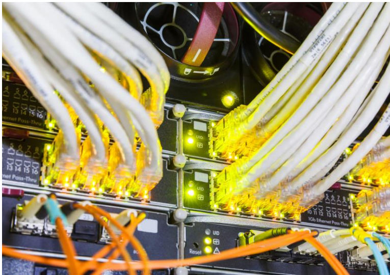
Figure 5: The rear of a heavily populated cabinet
